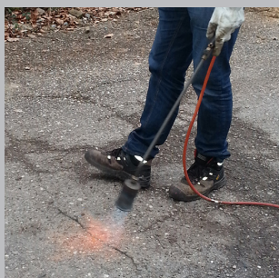
Brush away any dirt and remove moisture from the crack with a heat torch.
