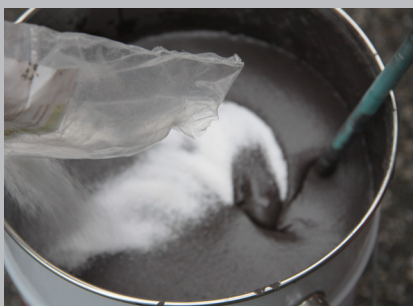
Combine the two components (ColdFill + hardener) using a drill with paddle attachment.
