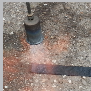
Bond BandFill to the crack by heating the material with a heat torch.
