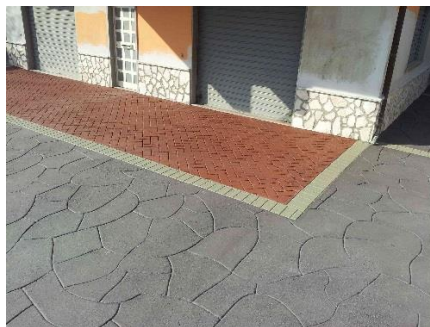
Designing of a private courtyard: application of AquaRoute™ Deco Rough on stamped asphalt (red, grey and light grey area)
